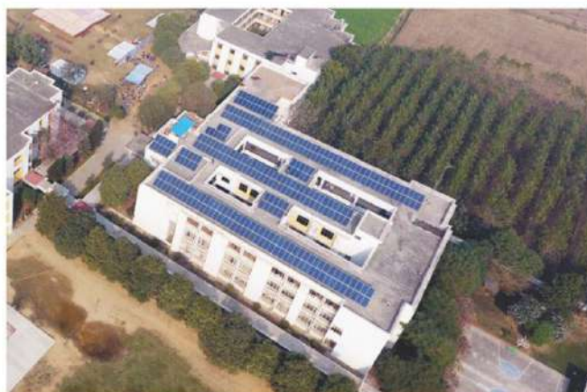
Energy-Saved-Solar Plant - 150 KW
